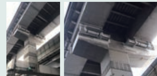
Photo 6. Bridges equipped with friction dampers (Route 11 Daiba Line)
