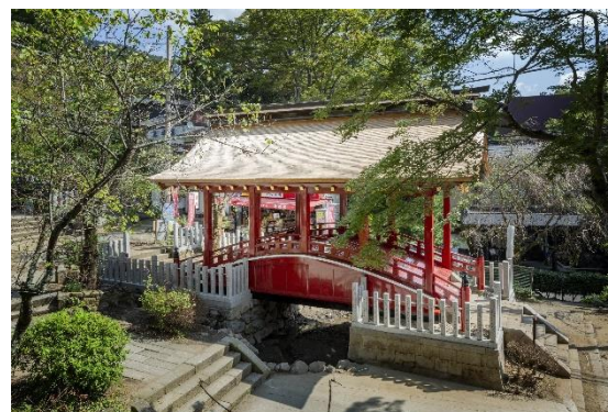
Kongo Gumi (Tsukuba, Ibaraki) Tsukubasan Shrine Shinkyo Bridge (cultural asset designated by Ibaraki) repair work
