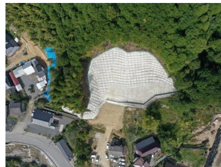
Toko Geotech Miyazono District emergency steep sloping land collapse prevention work at site 1
