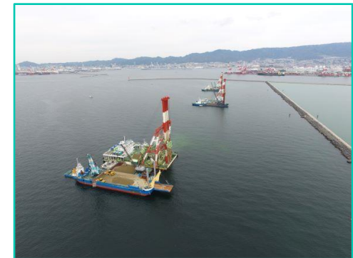
Ground reinforcement work on facilities adjoining the fairway at the Port of Kobe
