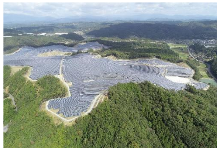
Asunaro Aoki Construction Pacifico Energy Sakuto Mega-Solar Power Plant construction site preparation (A and G blocks)
