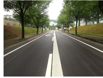
Niigata Mirai Construction Maintenance and repair No. 2 Harashinden Kosaka Line Pavement replacement work
