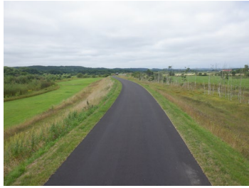
Asunaro Road Kushiro River repair work Isobunnai Top edge protection work outside the embankment
