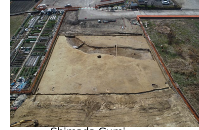
Shimada Gumi 4-chome, Shindo, Matsubara-shi Land readjustment project Archaeological excavation of buried cultural properties
